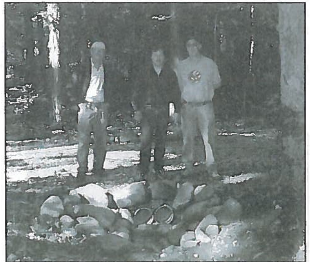
Superintendent Mike Walter, Asst. Superintendent. Paul Konwerski, Jr. and Nate Case on new gravel over PVC drains
